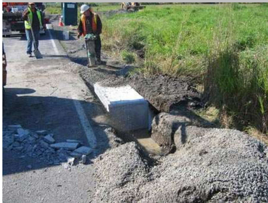
Qwest contractors installing phone cable splice box to reroute Qwest phone cable This took several men and several large machines 3 days work. The work crew had no idea why they were doing it. The City of Enumclaw has to also reroute a water line.
