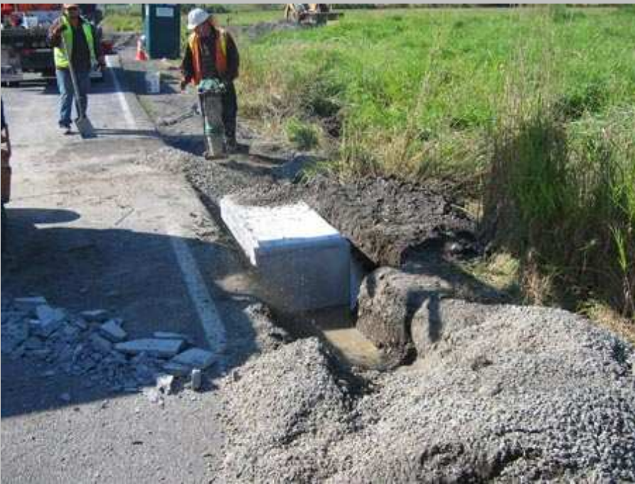
Qwest contractors installing phone cable splice box to reroute Qwest phone cable This took several men and several large machines 3 days work. The work crew had no idea why they were doing it. The City of Enumclaw has to also reroute a water line.
